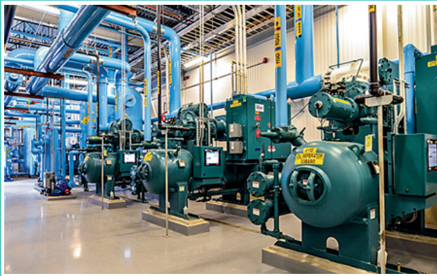
Figure 4: Well-designed and maintained refrigeration plant
